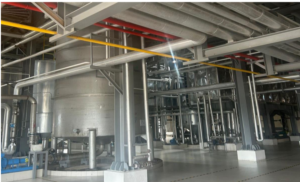
Figure 15. STAOF refinery installation
